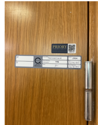
Fire Door Certification label.
