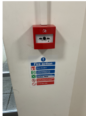
Fire Action Notice and Manual Call Point.
