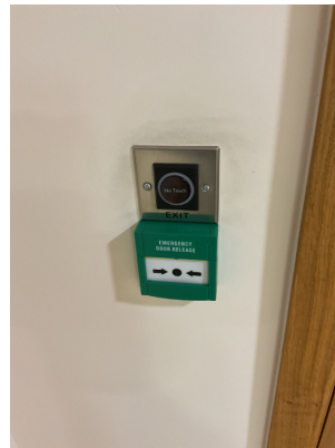
Exit and Emergency door release.
