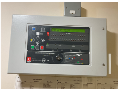
Main Fire Alarm Panel
