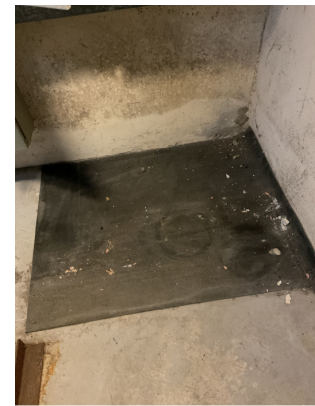
Rubber matting plant room.
